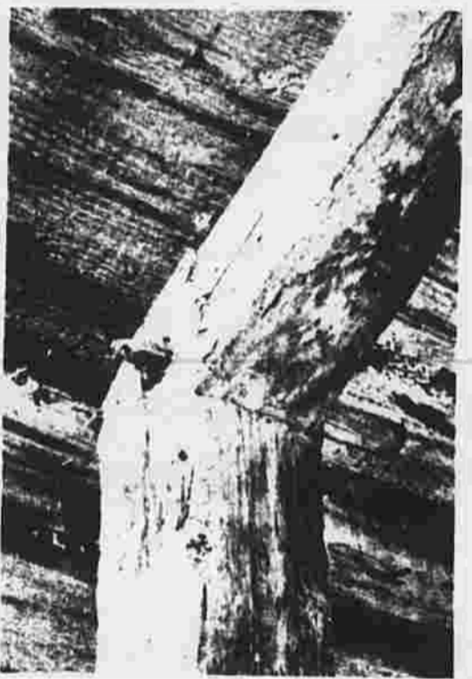
The tool is used to drive in trunnels (trenails), such as the one we see here holding roof timbers together.
